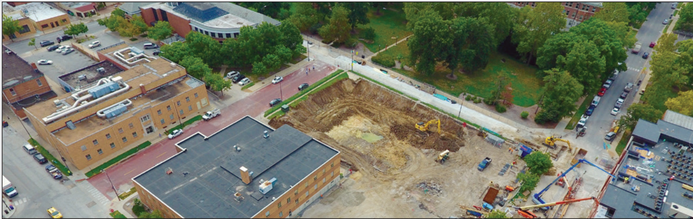
Site work has begun on the Center for Missouri Studies, the State Historical Society of Missouri's new Columbia headquarters building at the corner of Sixth and Elm Streets. The project is scheduled for completion in the spring of 2019. Learn more on the Society's website at shsmo.org/thecenter .
